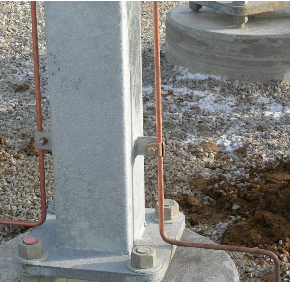
Substation earthing riser
