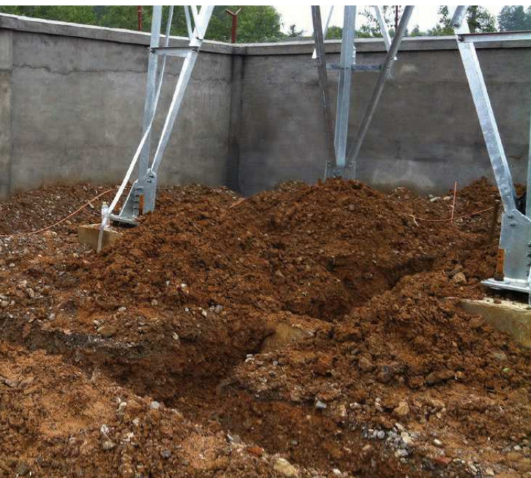
Telecom tower grounding
