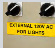
Equipment & Panel Labeling
