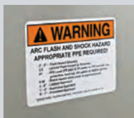
Arc Flash Labeling
