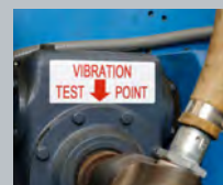
Lean / 5S Labeling
