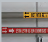
Pipe & Valve ID
